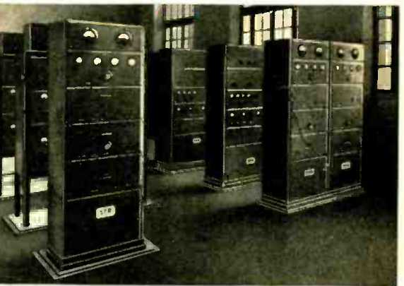
Above—A view of part of the system of elaborate filter circuits, built into panels, which are used to scramble or mix-up the speech frequencies, in order to prevent their being picked up by the average S-W listener.
